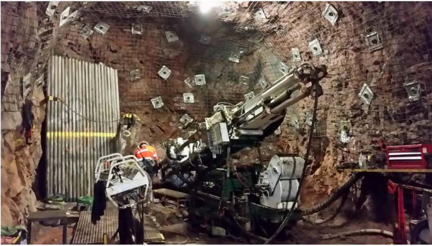
An underground drill program was carried out as part of the technical studies at the Mount Gordon site, now known as Capricorn Copper.
